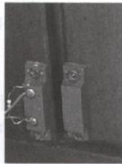
Figure 48. Magnetic switch on a sliding door.
