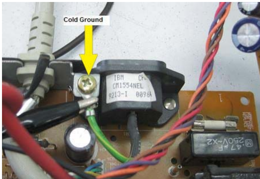
Figure 12.4- Connect The Scope Ground To Cold Ground If You Want To Check The Secondary Side
